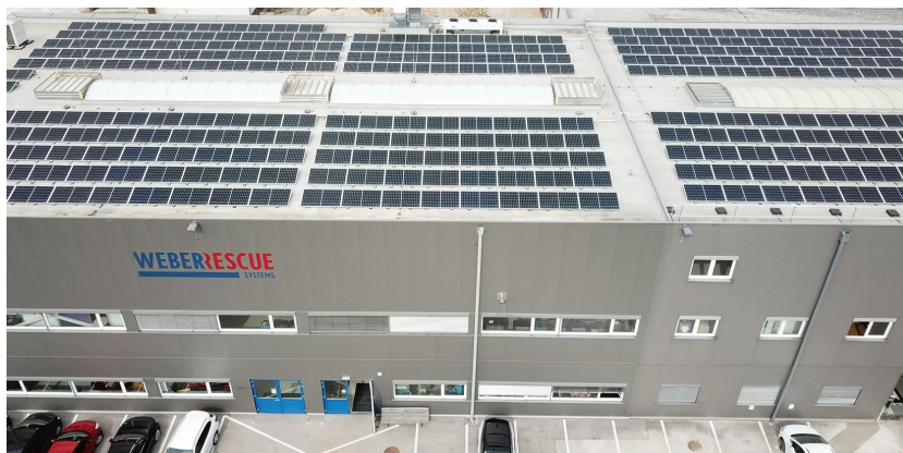
Photovoltaic plant with 364 kWp installed capacity
